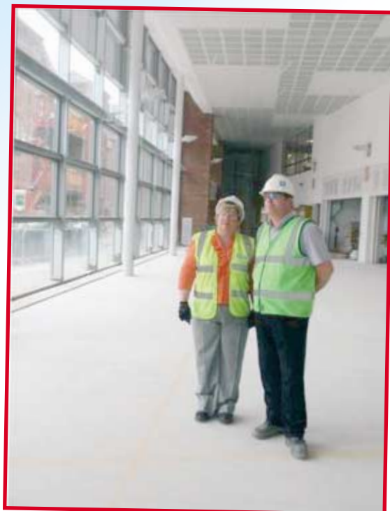
Ann Marr, Chief Executive with Jerry Daly, Project Manager from Taylor Woodrow in the main entrance of the new Whiston Hospital.
